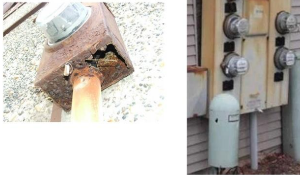
Figure 10 – Rusty, Damaged, Poorly-Mounted Meter Sockets.
