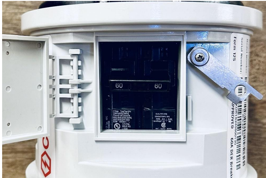
Figure 28 – Verify the PV/DER circuit breaker is open (OFF) on the bottom of the MSA Base.
