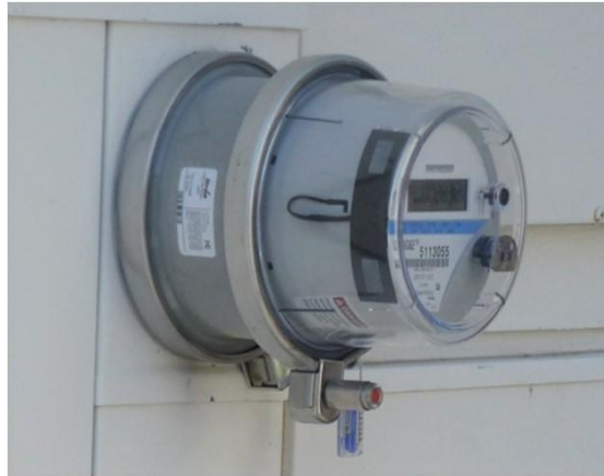
Figure 9 – Existing Meter and Meter Socket Adapter.
