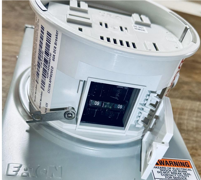
Figure 30 – Circuit Breaker Cover open on the bottom of the MSA Base.
