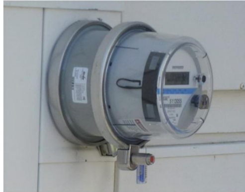
Figure 10. Existing Meter and Meter Socket Adapter.
