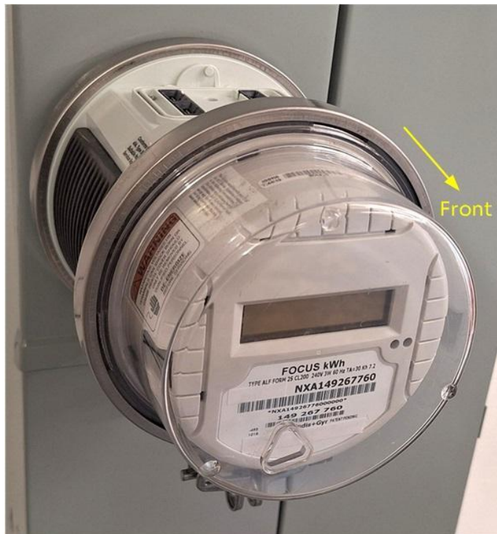
Figure 23. MSA Base with Utility Meter Installed.
