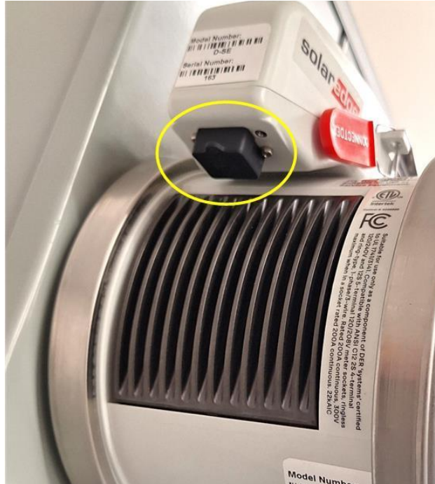
Figure 28. Ethernet RJ-45 Port Capped Off. IslandDER MSA ready for connection to BESS.
