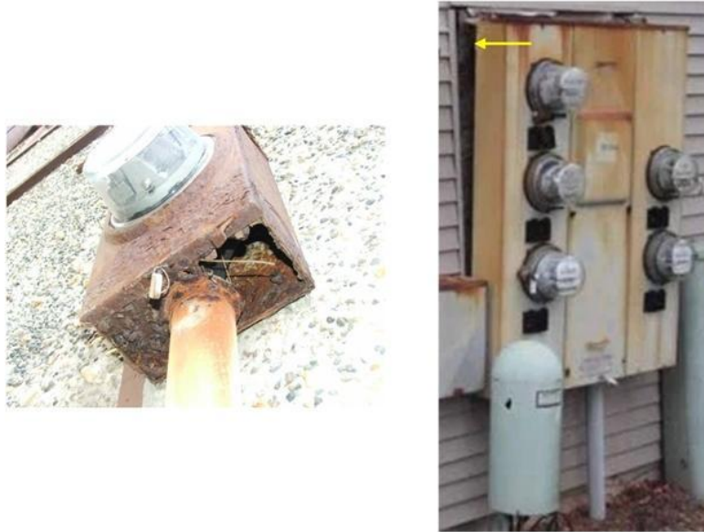
Figure 11. Rusty, Damaged, Poorly-Mounted Meter Sockets.
