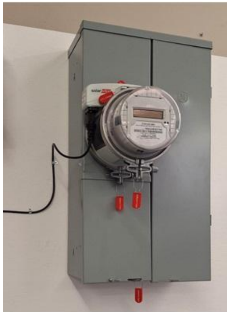
Figure 39. IslandDER Digital MSA. Ethernet cable routing towards the BESS.
