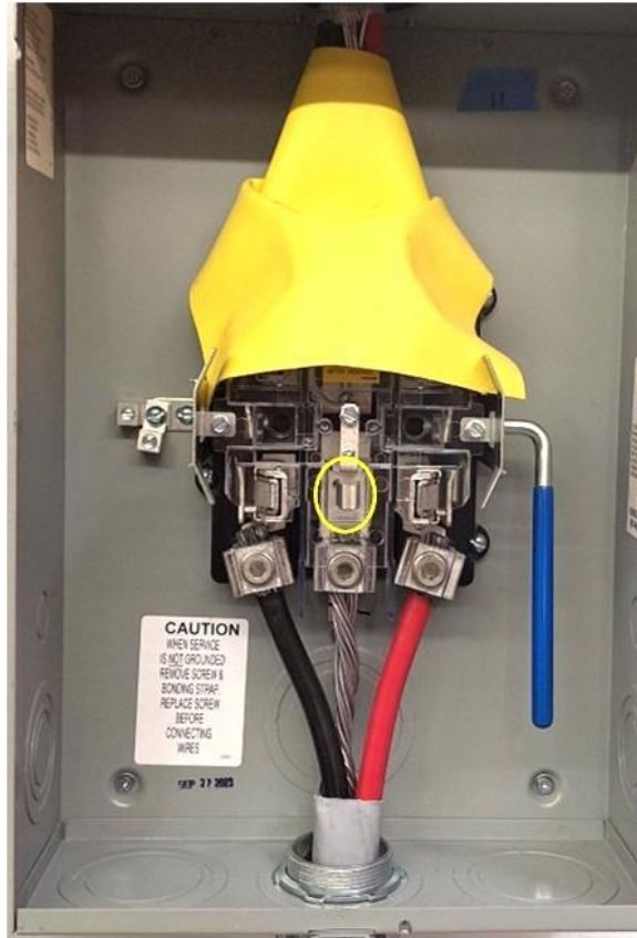
Figure 19. Meter socket with 5 th jaw at 6 o'clock.
