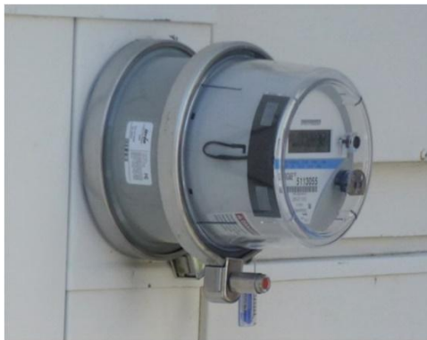
Figure 11 – Existing Meter and Meter Socket Adapter.
