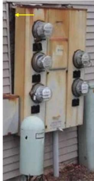
Figure 12 – Rusty, Damaged, Poorly-Mounted Meter Sockets.
