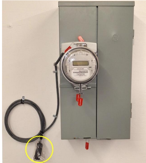
Figure 28 – IslandDER Analog Installed and Ready for 3 rd Party Integration.
