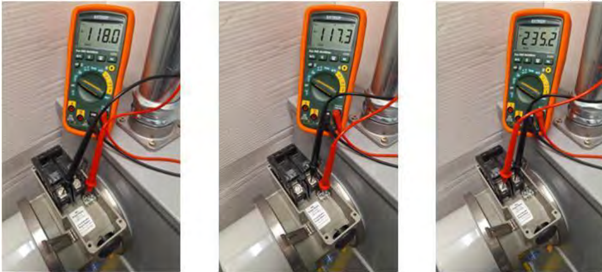
Figure 26 – Verify Voltage at Connection Module
