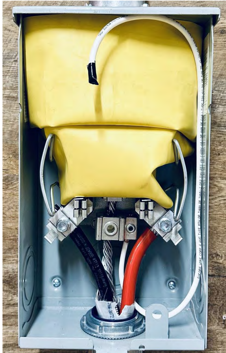
Figure 15 – Route the Neutral Within Meter Socket
