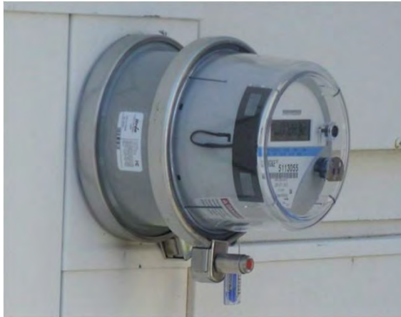
Figure 9 – Existing Meter and Meter Socket Adapter
