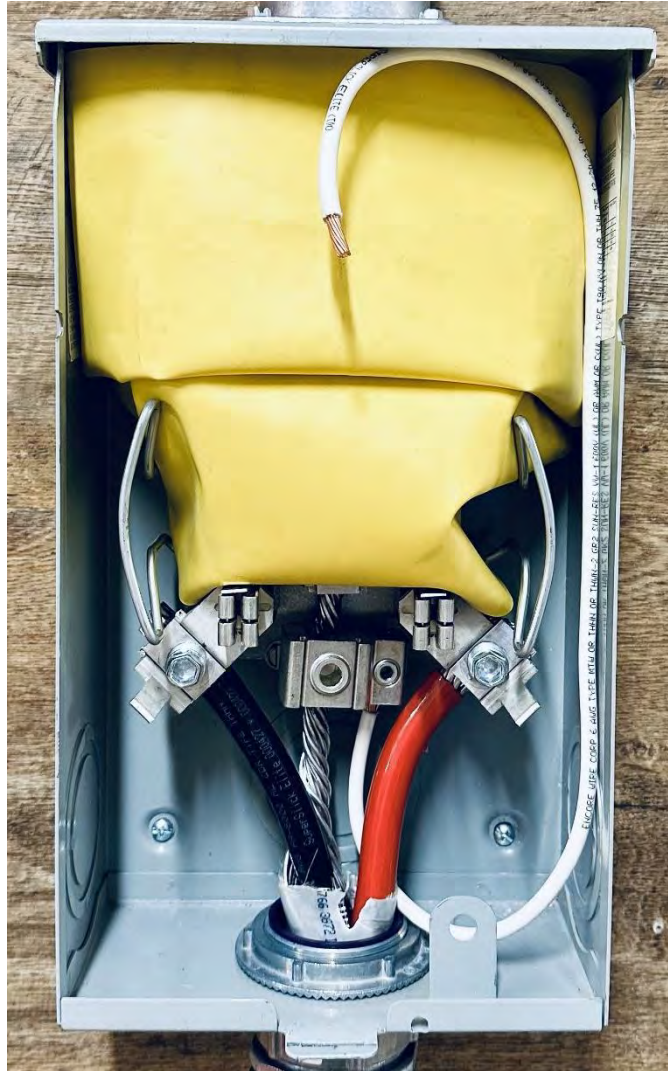
Figure 17–Neutral Ready for EV MSA Termination
