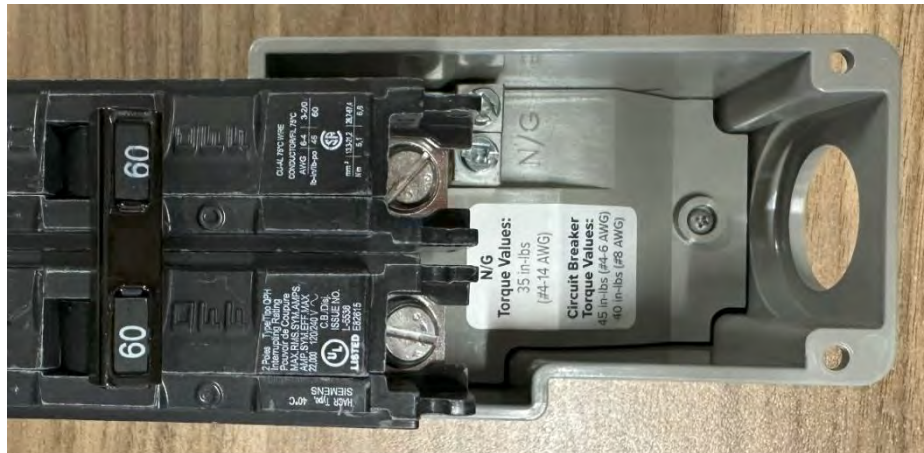
Figure 32 – Connection Module Terminals
