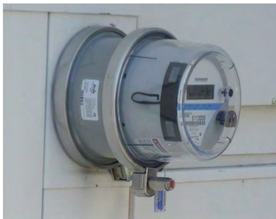
Figure 9 – Existing Meter and Meter Socket Adapter
