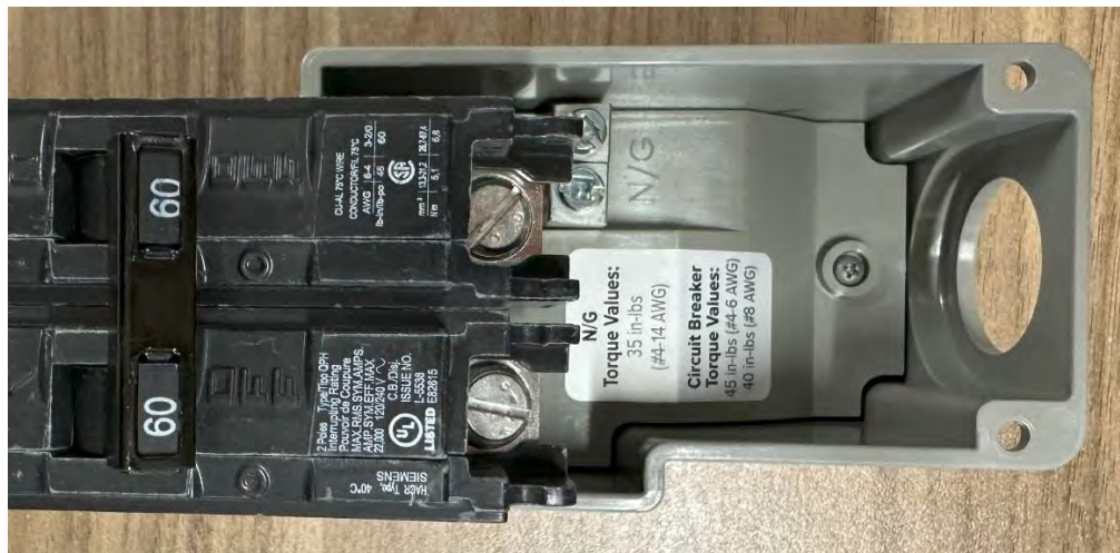
Figure 31 – Junction Box Terminals
