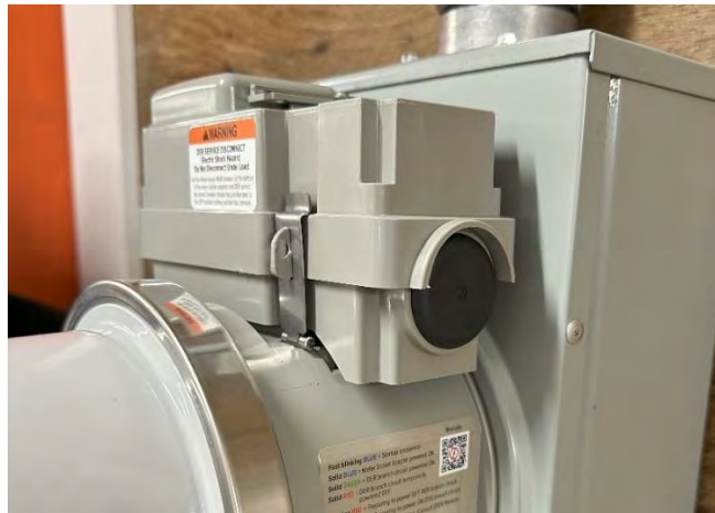
Figure 28 – Sealed Junction Box
