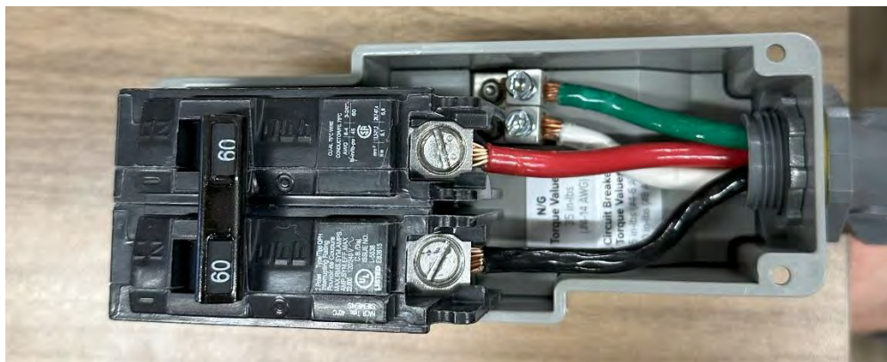
Figure 32 – Junction Box Wiring
