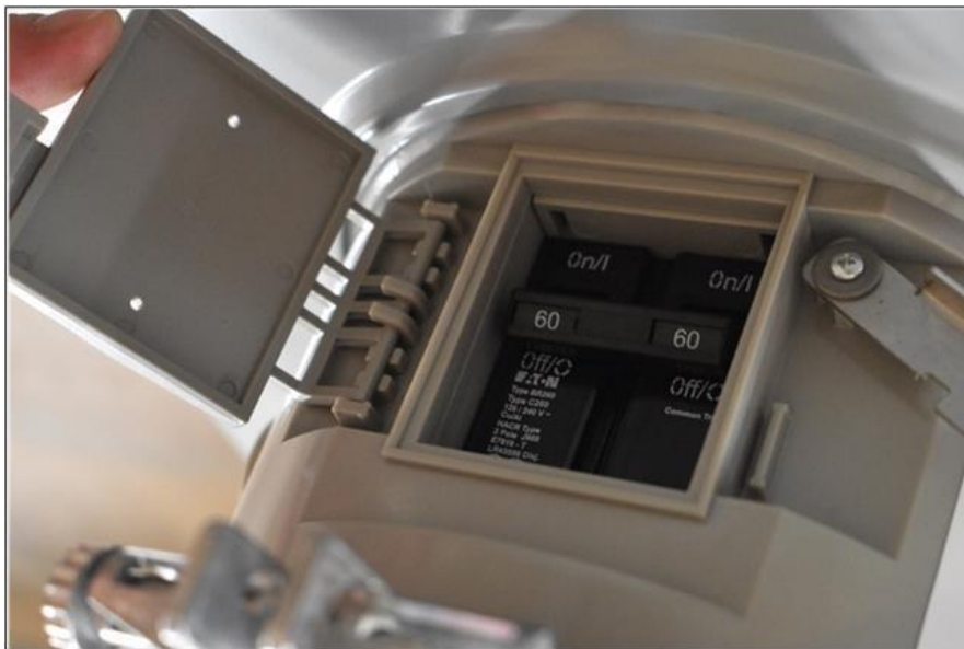
Figure 23 – Verify Solar Meter Adapter breaker is open (OFF)
