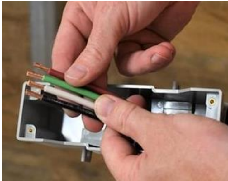
Figure 32 – Wiring at Junction Box
