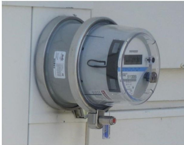
Figure 8 – Existing Meter and Socket Adapter
