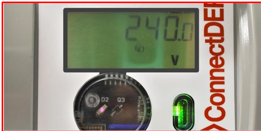
Figure 30 – Solar Meter Adapter + Smart Module Normal Status
