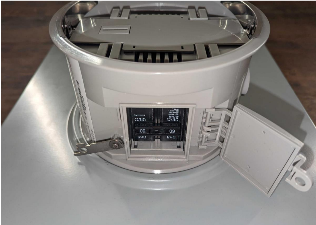
Figure 18 – Circuit Breaker Cover
