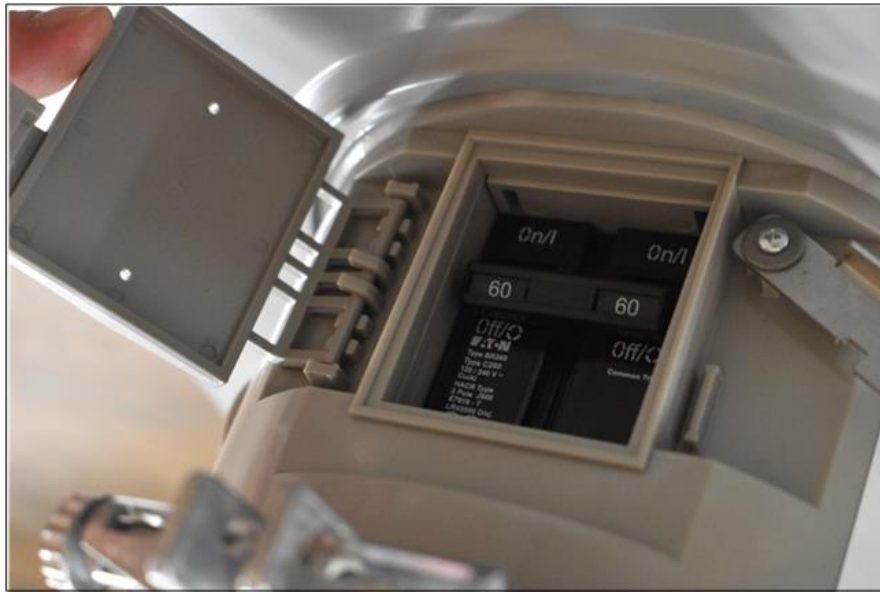
Figure 16 – Verify MSA breaker is open (OFF)
