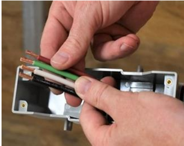
Figure 25 – Wiring at Junction Box
