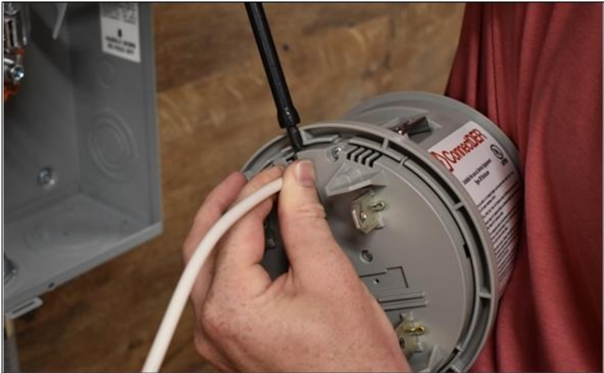
Figure 22 – Terminate the Neutral to Solar Collar
