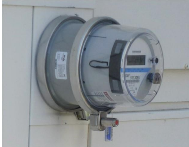
Figure 8 – Existing Meter and Socket Adapter
