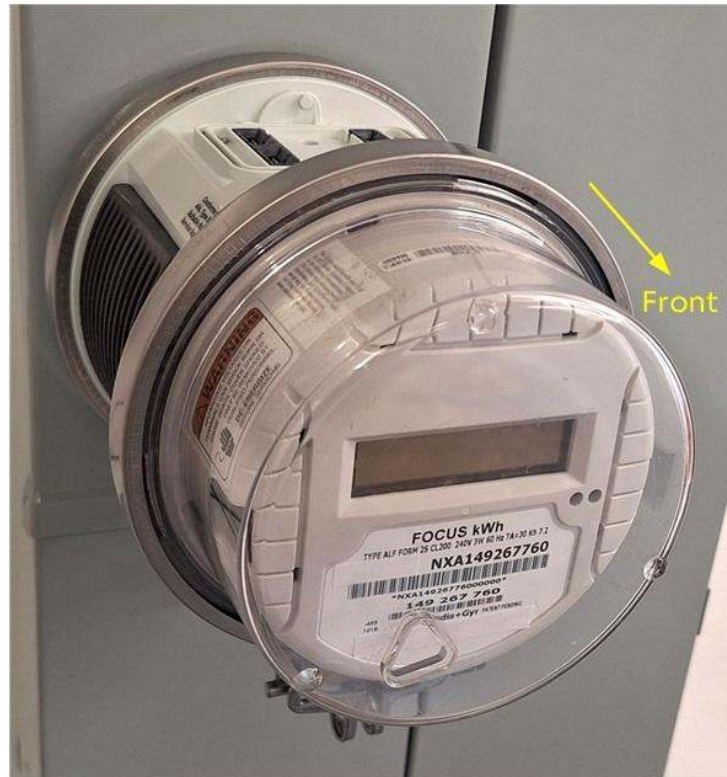
Figure 23. MSA Base with Utility Meter Installed.
