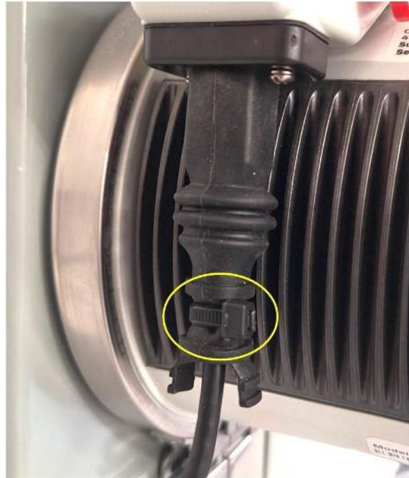
Figure 37. Cable Tie Around Boot and Grommet.
