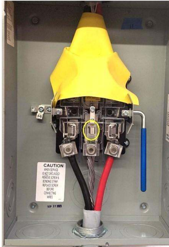
Figure 19. Meter socket with 5 th jaw at 6 o'clock.
