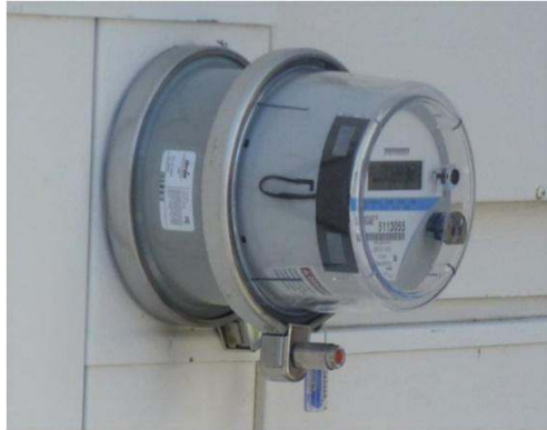
Figure 10. Existing Meter and Meter Socket Adapter.
