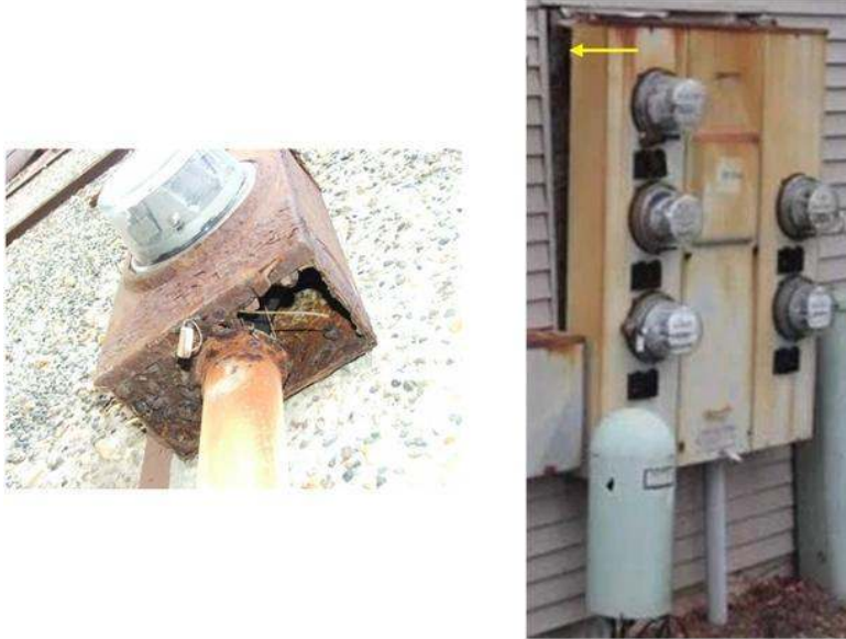
Figure 11. Rusty, Damaged, Poorly-Mounted Meter Sockets.
