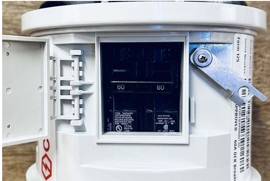
Figure 29. Verify the PV/DER circuit breaker is open (OFF) on the bottom of the MSA Base.
