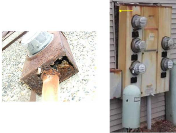
Figure 10. Rusty, Damaged, Poorly Mounted Meter Sockets.
