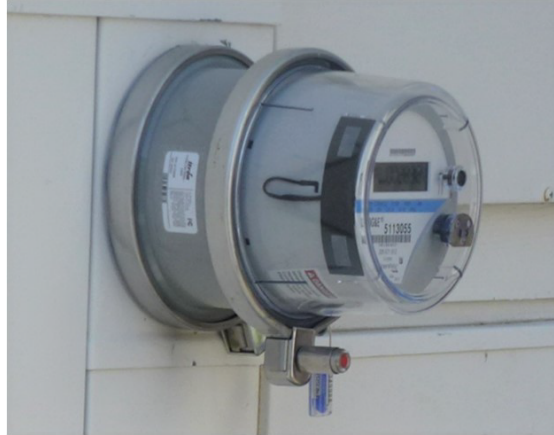
Figure 9. Existing Meter and Meter Socket Adapter.
