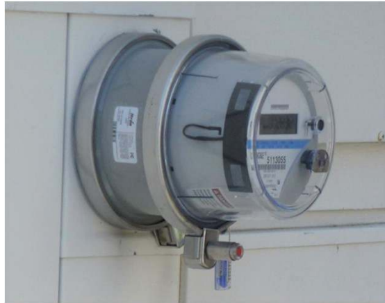
Figure 9. Existing Meter and Meter Socket Adapter.
