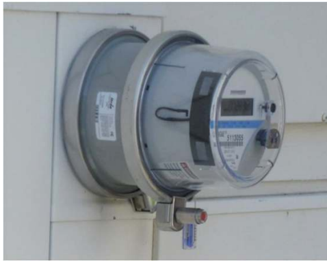
Figure 10. Existing Meter and Meter Socket Adapter.
