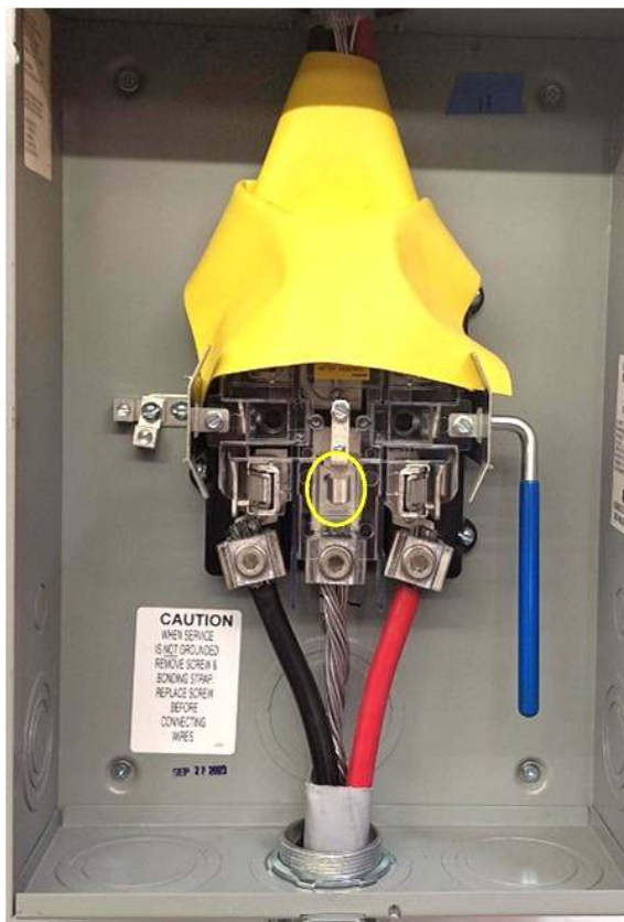
Figure 19. Meter socket with 5 th jaw at 6 o'clock.
