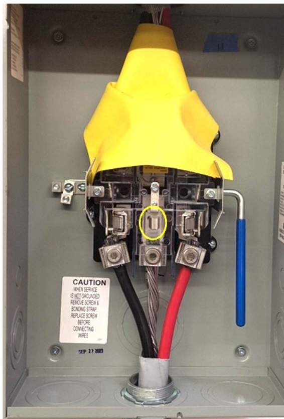
Figure 19. Meter socket with 5 th jaw at 6 o'clock.
