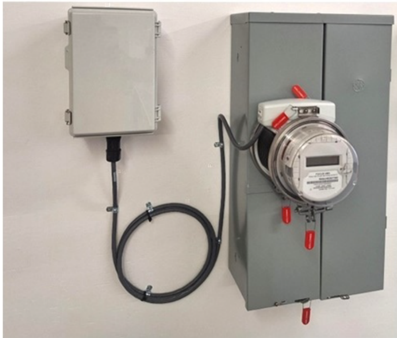
Figure 36. IslandDER MSA with the Communications Cable routed to the 3 rd Party DER System.
