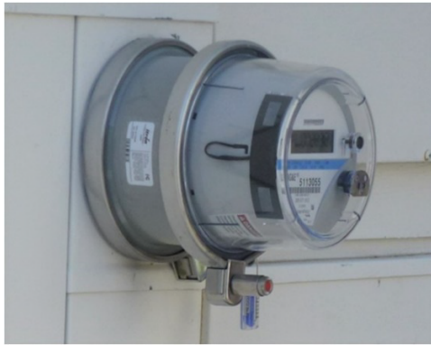
Figure 10. Existing Meter and Meter Socket Adapter.
