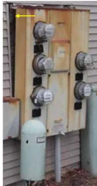
Figure 11. Rusty, Damaged, Poorly-Mounted Meter Sockets.
