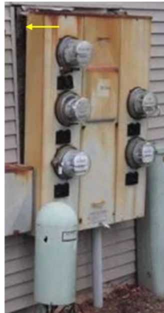
Figure 11. Rusty, Damaged, Poorly-Mounted Meter Sockets.
