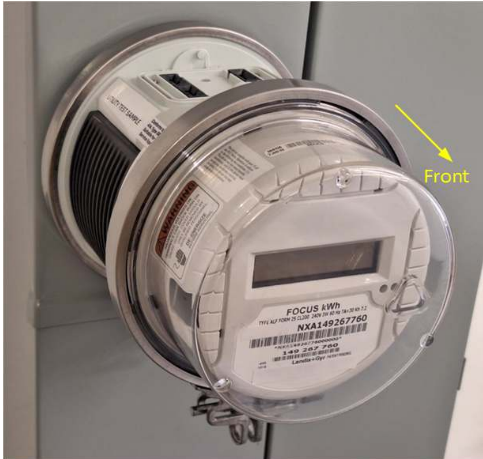
Figure 23. MSA Base with Utility Meter Installed.
